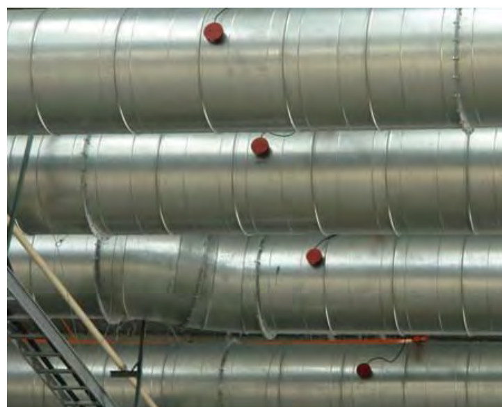
Spark Detectors Applied to an Array of Horizontal Ducting
